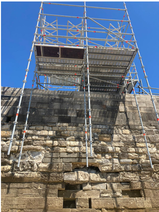
Figure 1: Clearly showing the damage to the sea wall and the Layher system scaffolding
